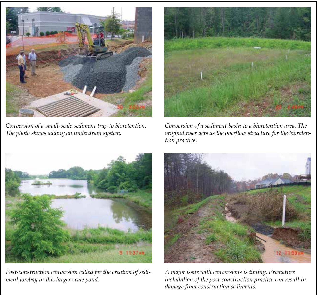
Figure E.3-1. Examples of E&S control practice conversions to post-construction BMPs (Photos: Center for Watershed Protection)
