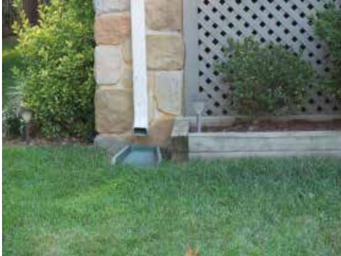
Figure 4.7-1. Simple Rooftop Disconnection (Photo: Center for Watershed Protection)
