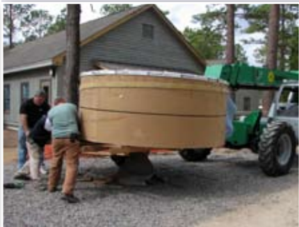
The tank arrives and is carried to an opening left in the building for this purpose.
